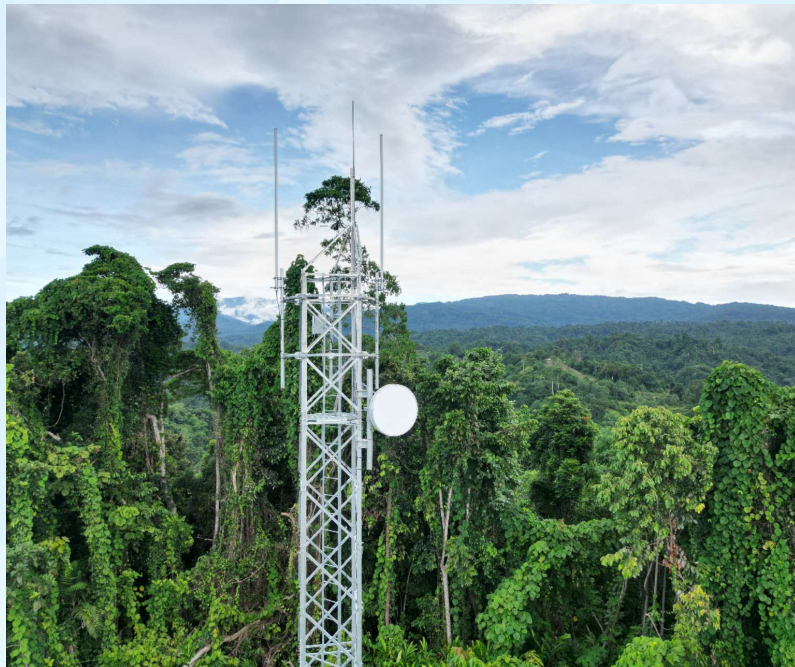
Telecommunication tower for the Solomon Islands National Broadband Network Project
