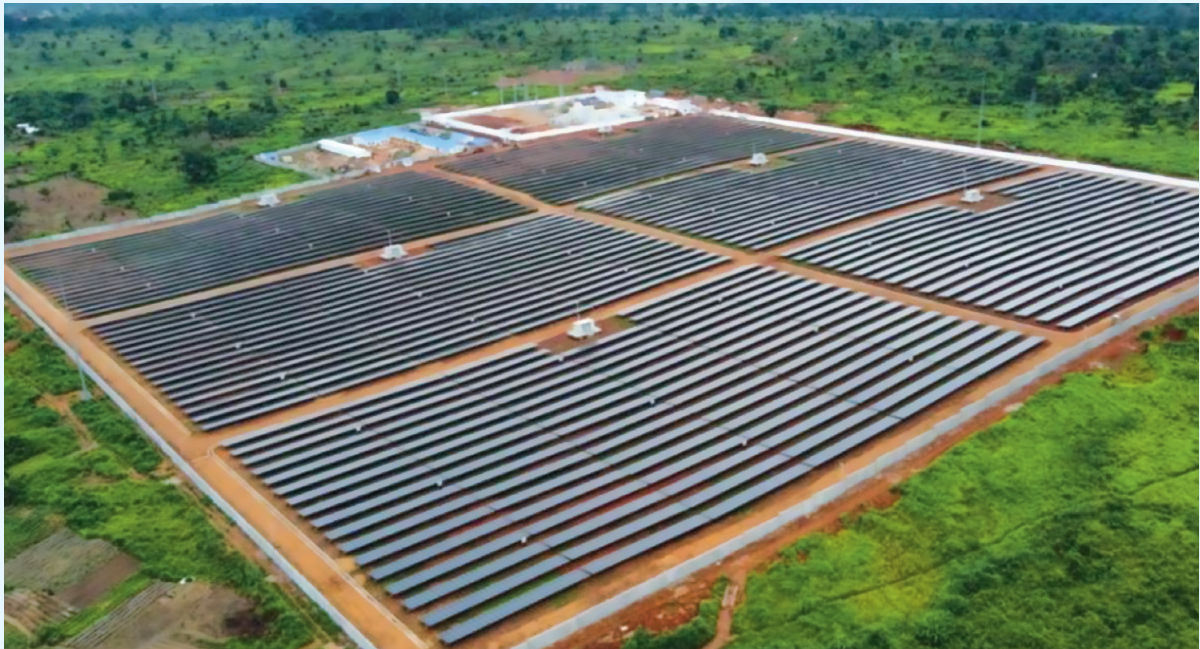
Sakai Photovoltaic Power Plant in the Central African Republic
