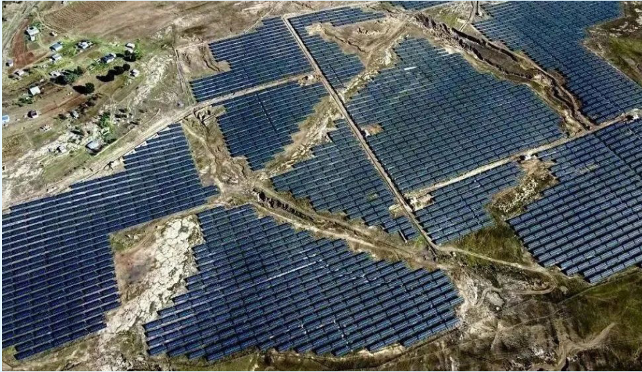
The 30 MW plant of the first phase of Mafeteng photovoltaic power station in Lesotho is completed
